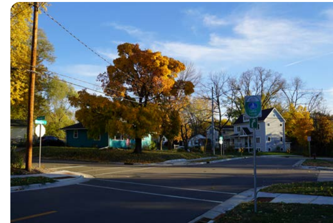
Five streets previously intersected at a single point. The reconstructed corridor now includes clear pavement markings, accessible curb ramps, and improved sightlines.
